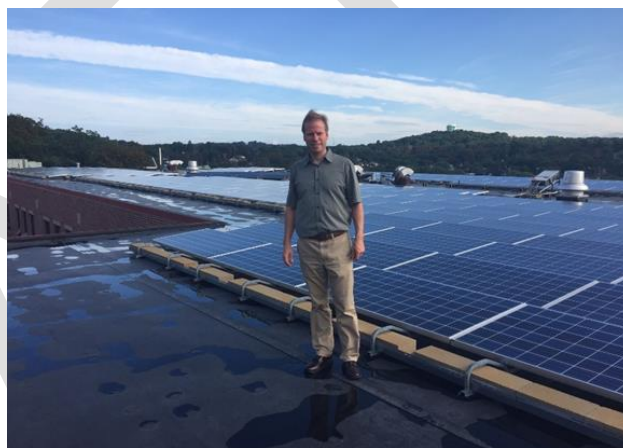
Solar array, Ottoson Middle School
