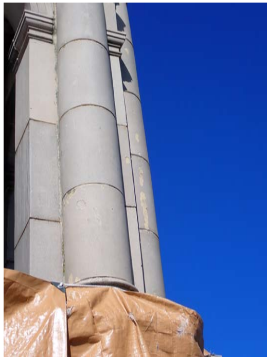
Figure 2. Terra cotta typical conditions with glaze loss.
