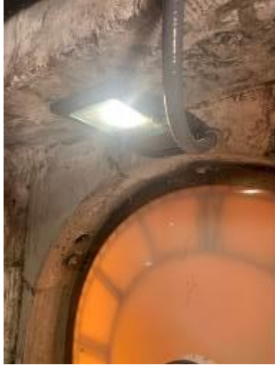
Light Fixture Upper Tower
