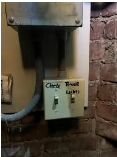
Switch Control in Lower Tower
