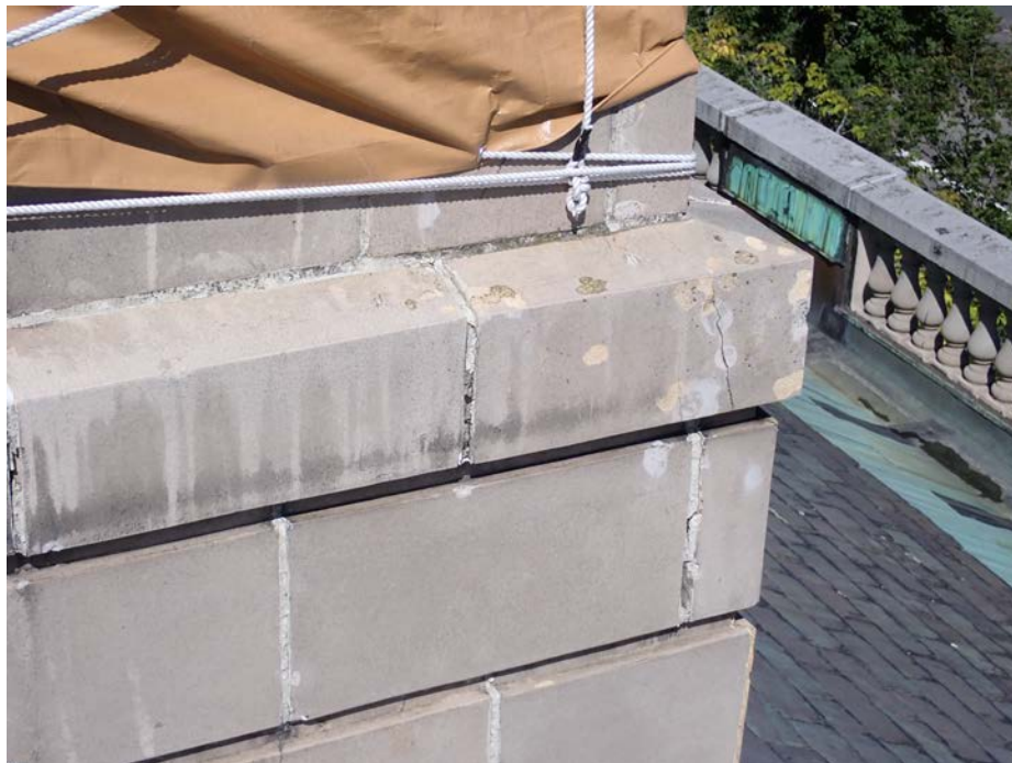
Figure 4. Lower podium at front of cupola showing mortar failure, glaze failure and crack through terra cotta.
