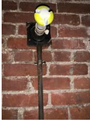
Light Fixture Lower Tower
