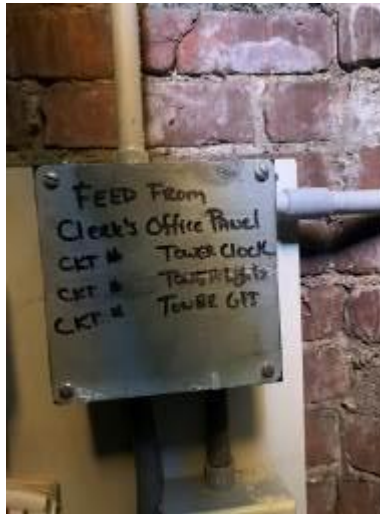
Junction Box Below Clock Tower
