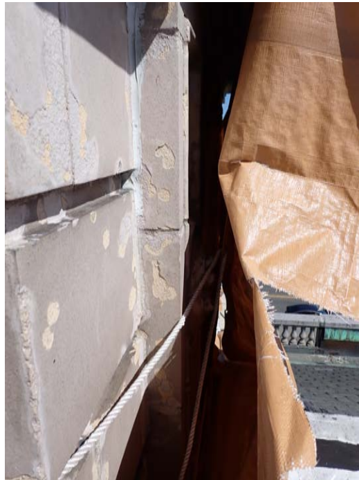
Figure 3. Podium level behind tarp showing extensive glaze failure.
